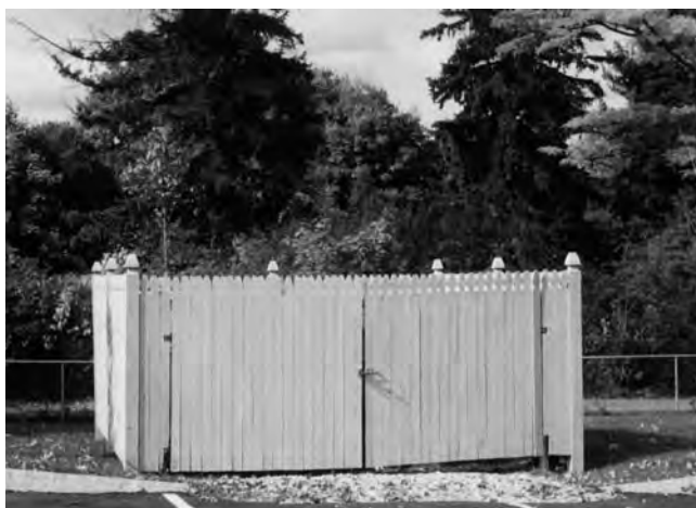
A typical trash enclosure. Its appearance could be improved by plantings along its sides, detailing to match nearby buildings, reinforcing the gates, and staining a dark color.
