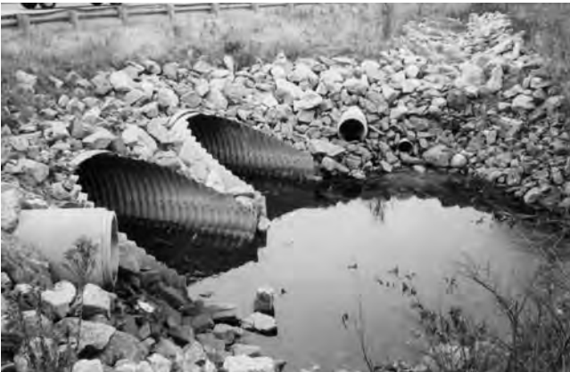
Rip-rap is often necessary to control erosion and stabilize slopes. In highly visible areas, a more refined appearance – accomplished through the use of handplaced stone and/or ground cover – is necessary to avoid situations such as this.
