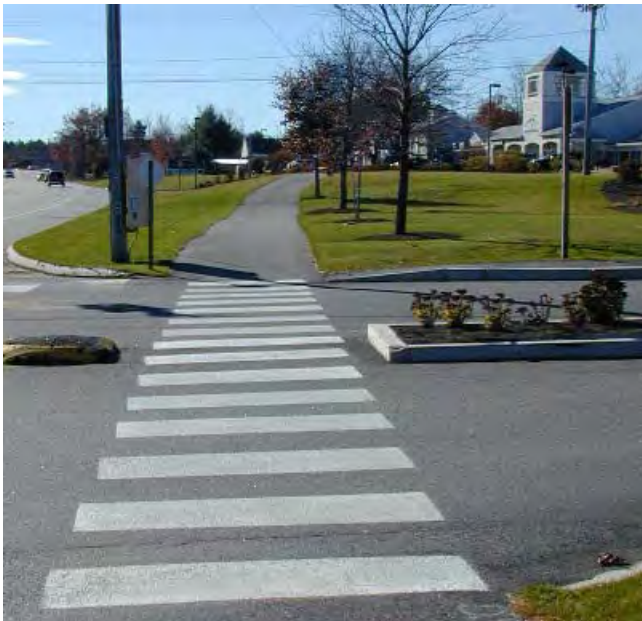
An island provides a refuge zone for pedestrians crossing this wide driveway. Permanent crosswalks should have been used to minimize annual maintenance.
