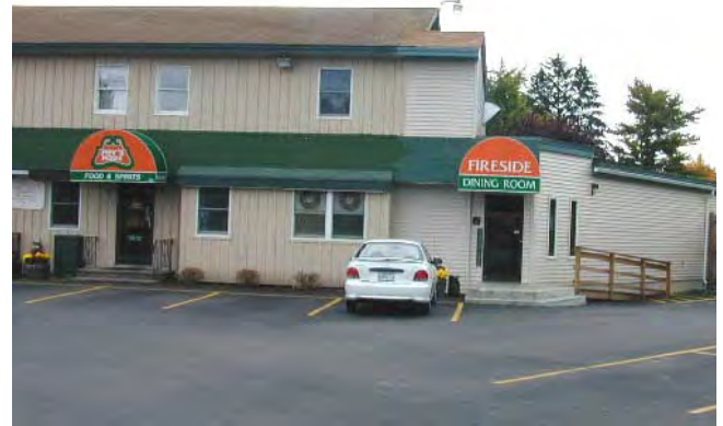
The addition to this restaurant does not relate to the form or building materials of the existing structure.
