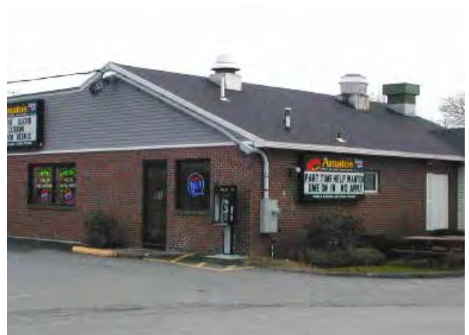
HVAC equipment and service connections are highly visible, adding unnecessary clutter to this small restaurant.
