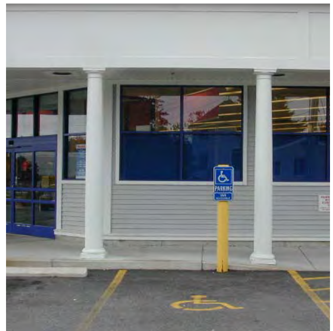
Details are critical to maintain long-term value. Plastic columns in this example are susceptible to snowplow damage. Bases are not flush with the pavement.
