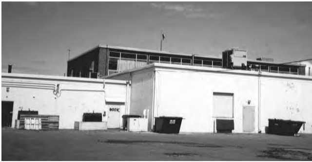
The roof-mounted mechanical equipment (as well as the dumpsters and downspouts) present an unsightly facade in a highly visible location.
