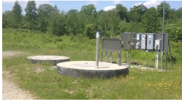
Sewer Pump Station on RT 26
