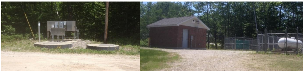
Sewer Pump Stations on RT 122
