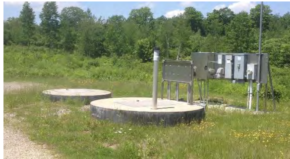
Sewer Pump Station on RT 26
