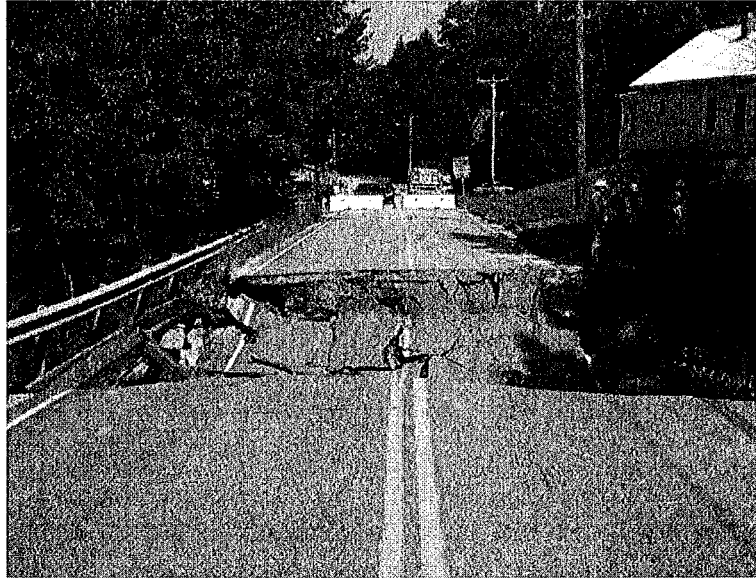
Bridge Collapse Minot, ME August 2008
