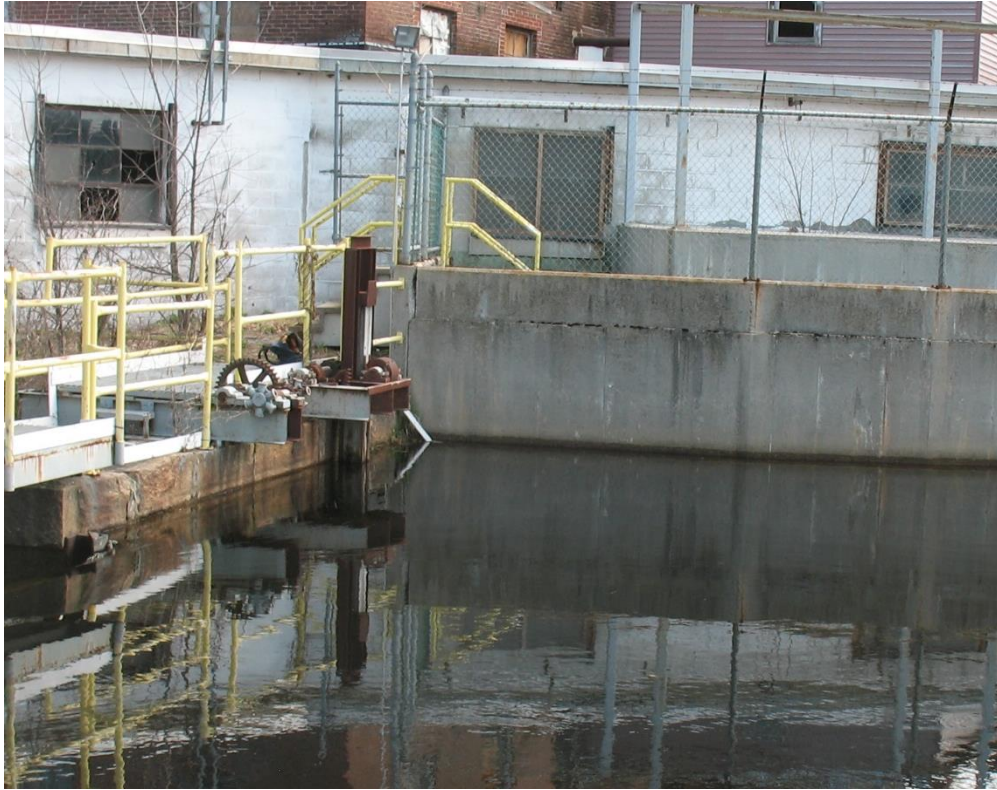
Photo 17. Upstream Face of Concrete Dam Section and Old Water Process Intake Gate Hoist.
