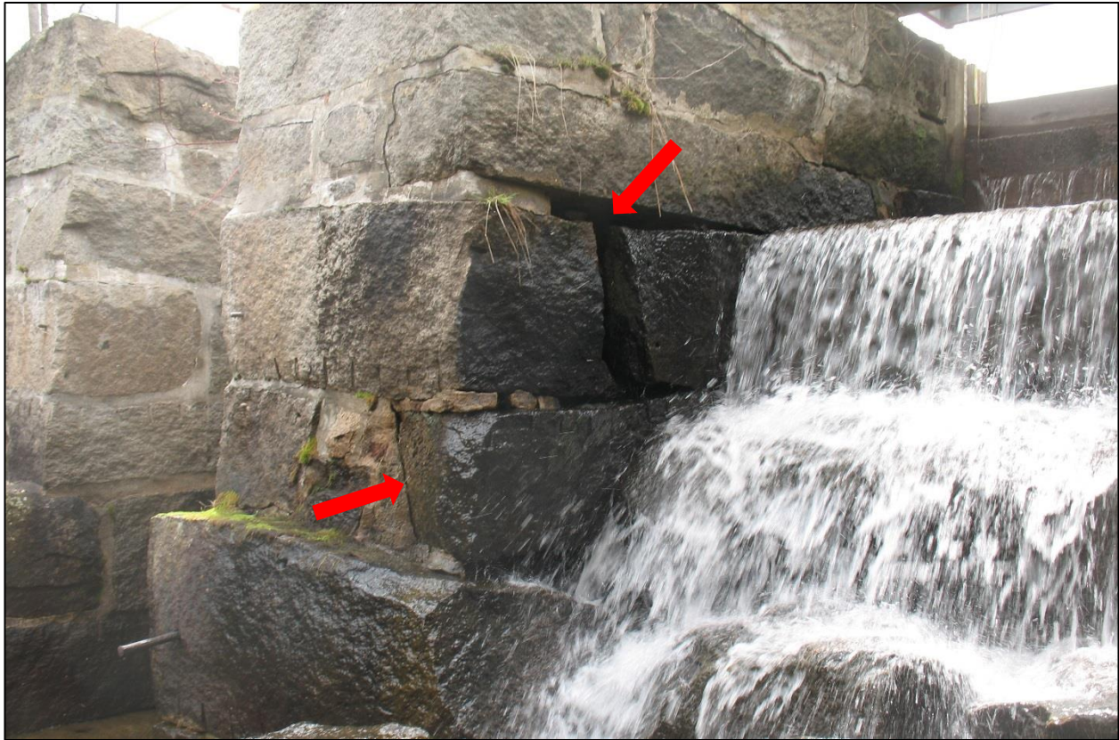
Photo 5. Right Wall of West Sluice. Note Missing Mortar, Large Voids and Crack in Masonry.
