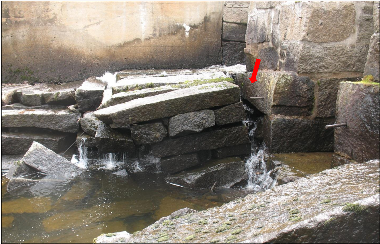
Photo 27. Movement and Separation of Stone Apron Block from Dam.
