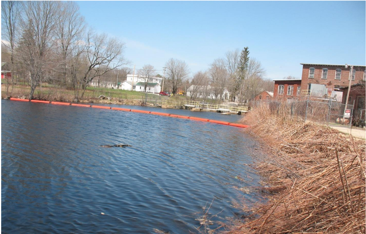
Photo 21. Log Boom in Approach Channel. Note Left Bank Trees and Right Bank Overgrowth.
