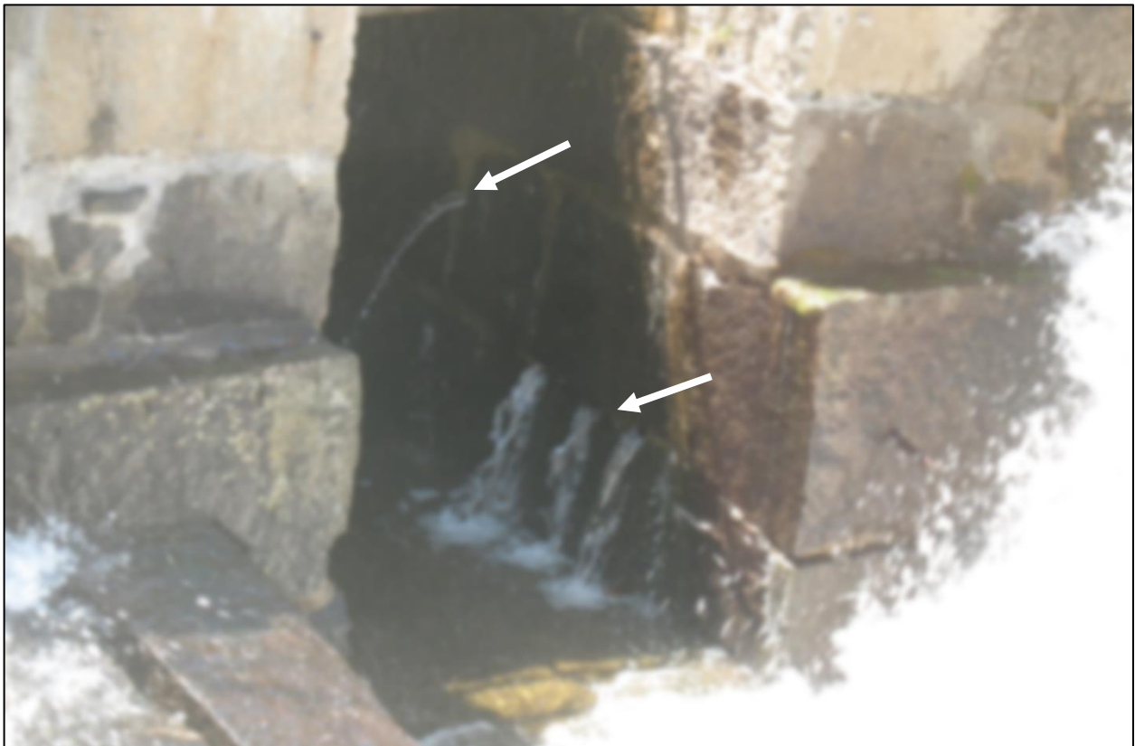
Photo 11. Downstream View of Central Sluice Masonry Leakage (arrows), 5/2/2018
