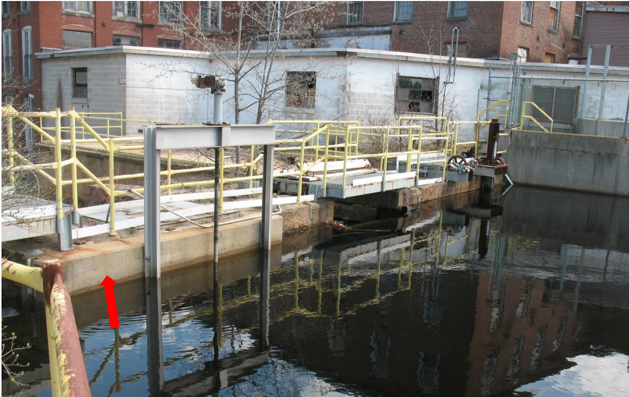
Photo 7. Upstream View of Central Sluice: Concrete Overlay (arrow), Gate Frame, Operator and Stem Installed in 1993.
