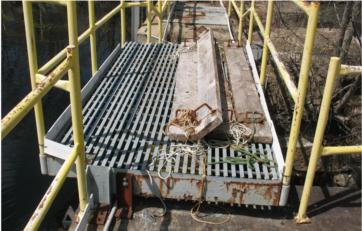
Photo 13. East Sluice Stoplog Operating Platform and Handrail. Note Steel Rust.
