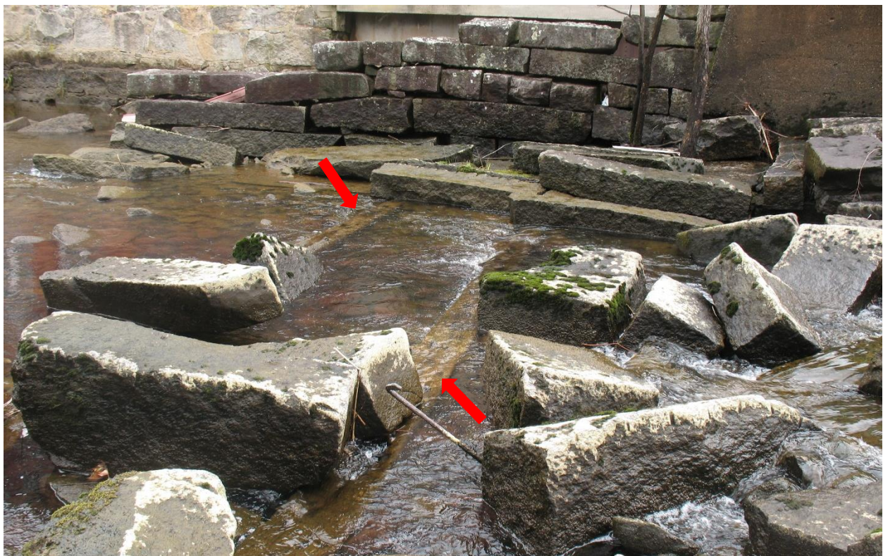
Photo 28. Exposed Base Timber Cribbing Used for Apron Construction.
