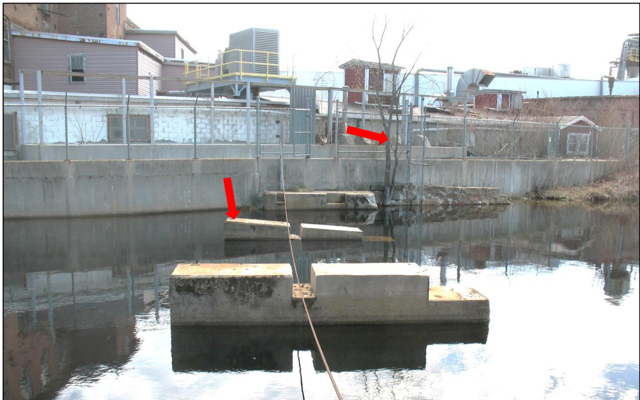
Photo 24. Right Approach Channel Retaining Wall and Old Piers Supporting Original Trashracks and Catwalk. Note Sagging Central Pier and Tree at Waterline.
