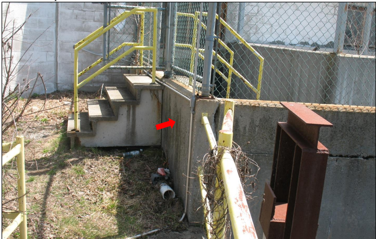
Photo 18. Concrete Dam Section at Mill Building and 3-foot High Concrete Parapet Wall (arrow) on Top of Dam.
