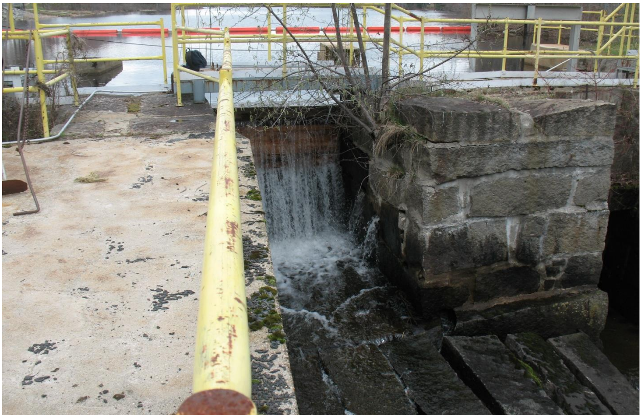
Photo 14. Downstream View of East Sluice. Note Leaking Stoplogs and Trees in Masonry.
