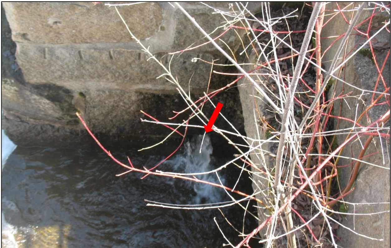
Photo 10. Central Sluice: Significant Right Wall Leakage near Sluice Bottom, Vegetation.
