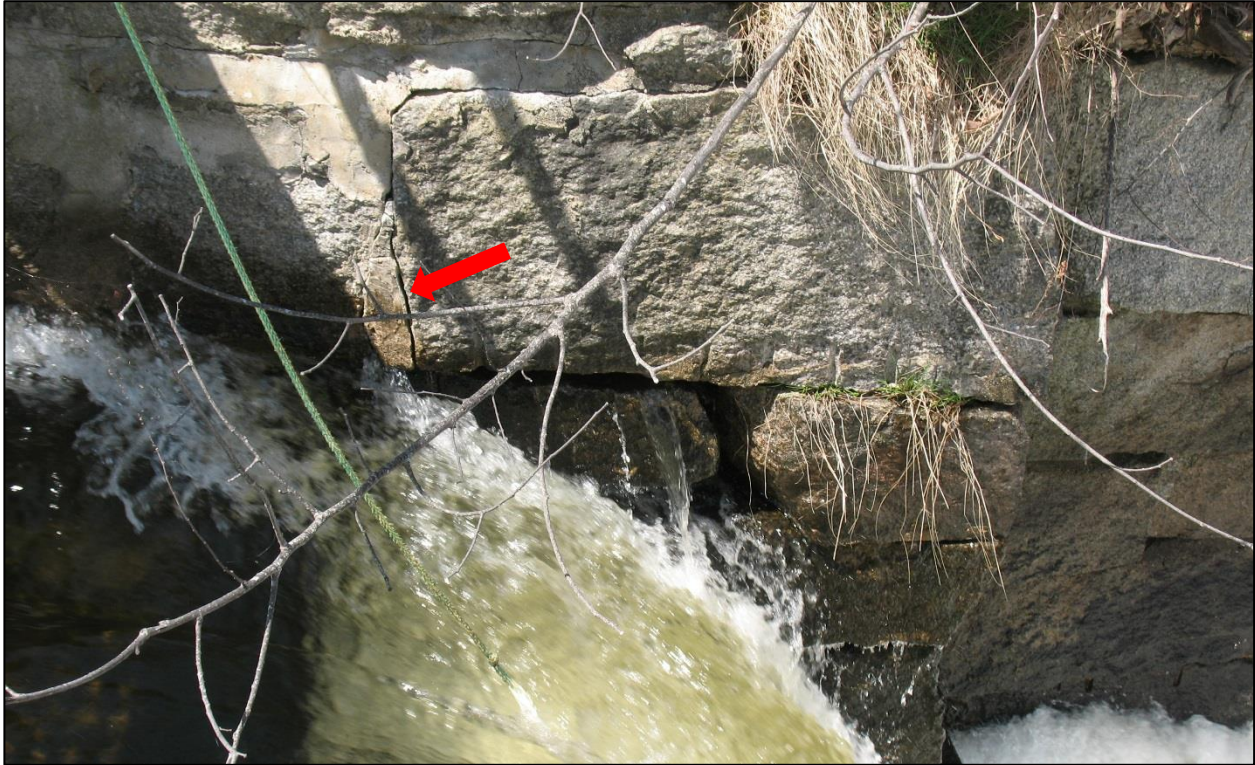
Photo 3. Left Wall of West Sluice. Note Open Joints, Crack in Masonry, Vegetation.
