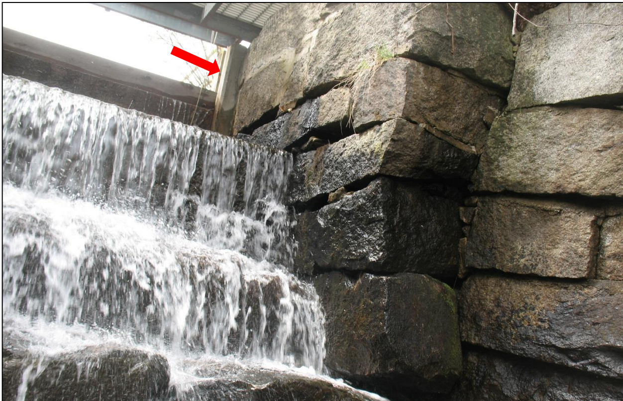
Photo 4. Downstream View of West Sluice: Voids in Masonry, Leaking Stoplogs, 1993 Concrete Overlay (arrow) in Sluice Opening.
