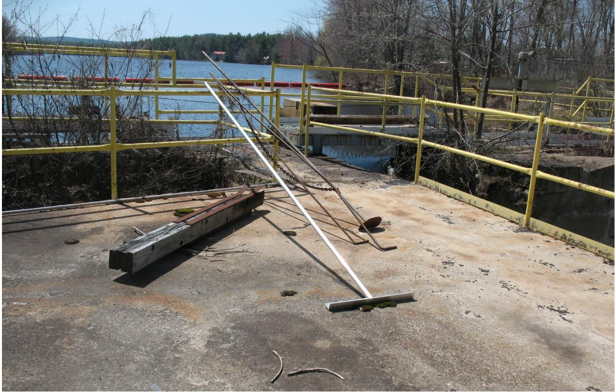
Photo 19. Concrete Dam Section Looking Upstream. Note Stored Lifting Rods Used for Stoplog Operation.
