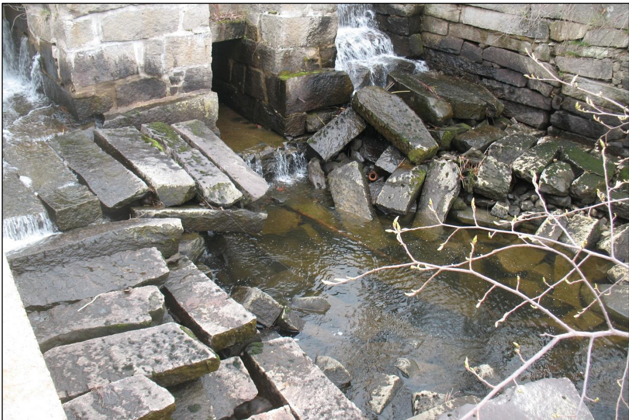
Photo 26. Disintegrated Stone Apron. Note Scour Hole at Dam Toe and in Channel Floor.
