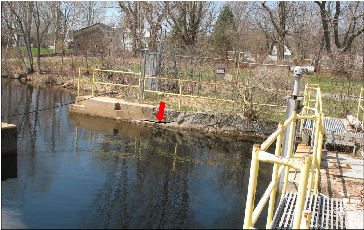
Photo 23. Left Approach Channel Retaining Wall. Note Wall Erosion and Large Crack at Waterline.
