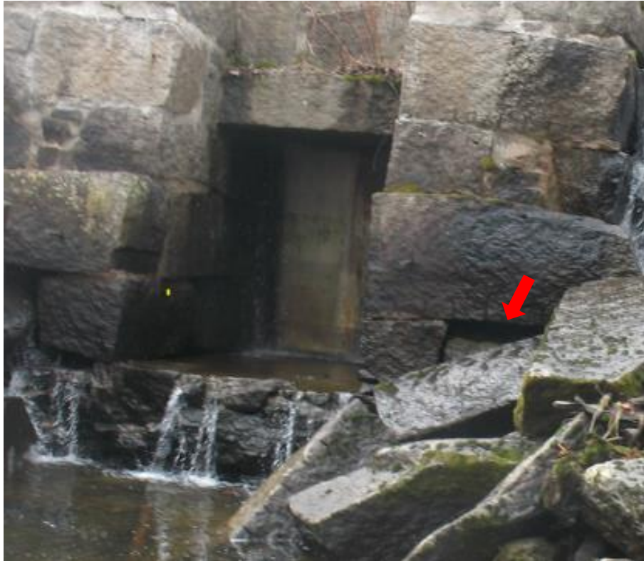
Photo 11. Downstream View of Closed Central Sluice Gate. Note Large Void in Masonry.
