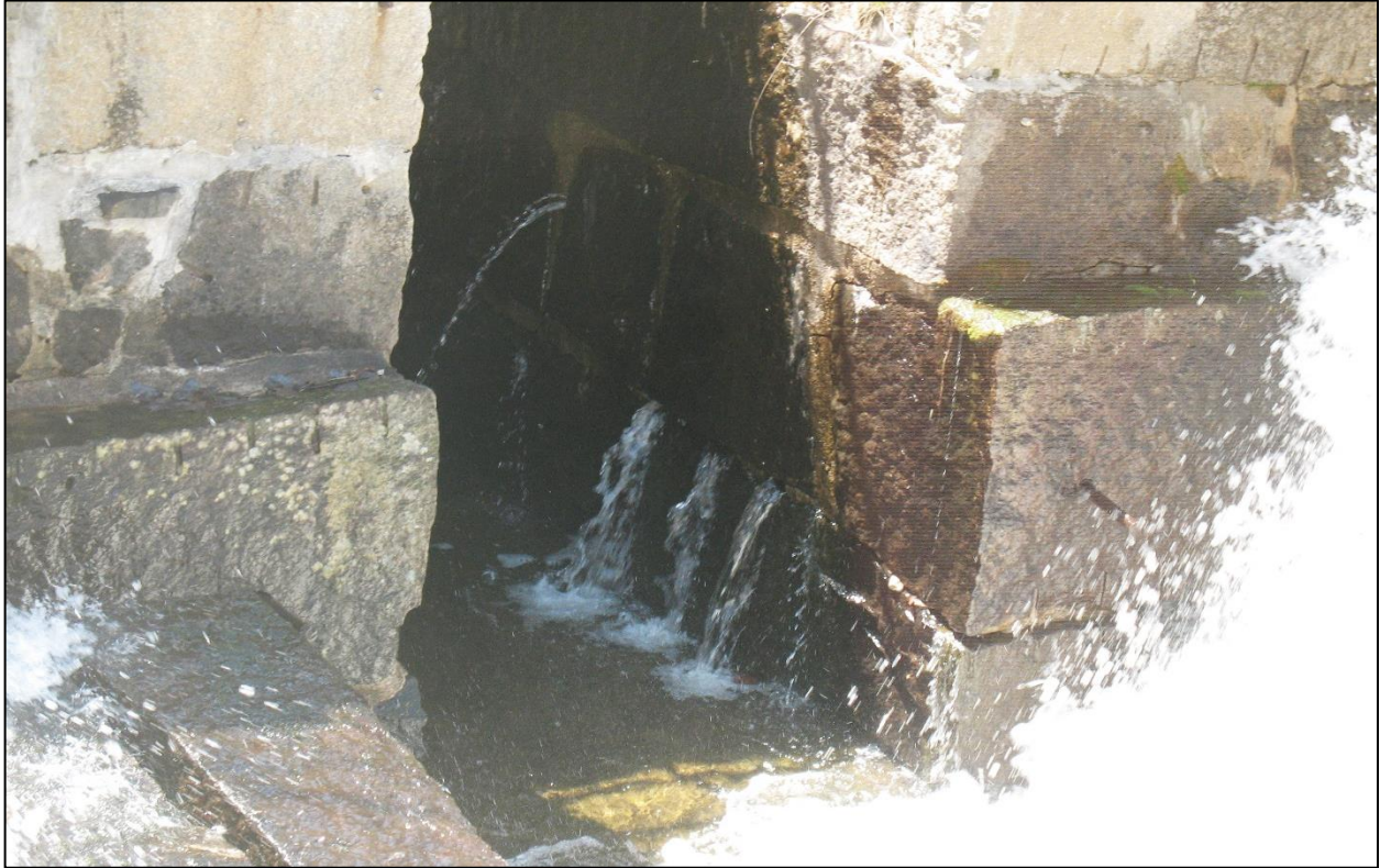
Photo 9. Downstream View of Central Sluice. Note Leakage in Left Wall.
